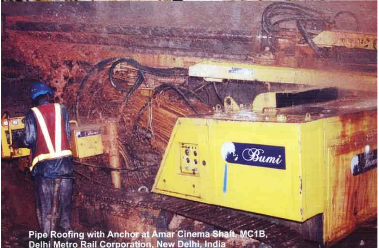
Anchors installed 8° upwards with high water ingress
