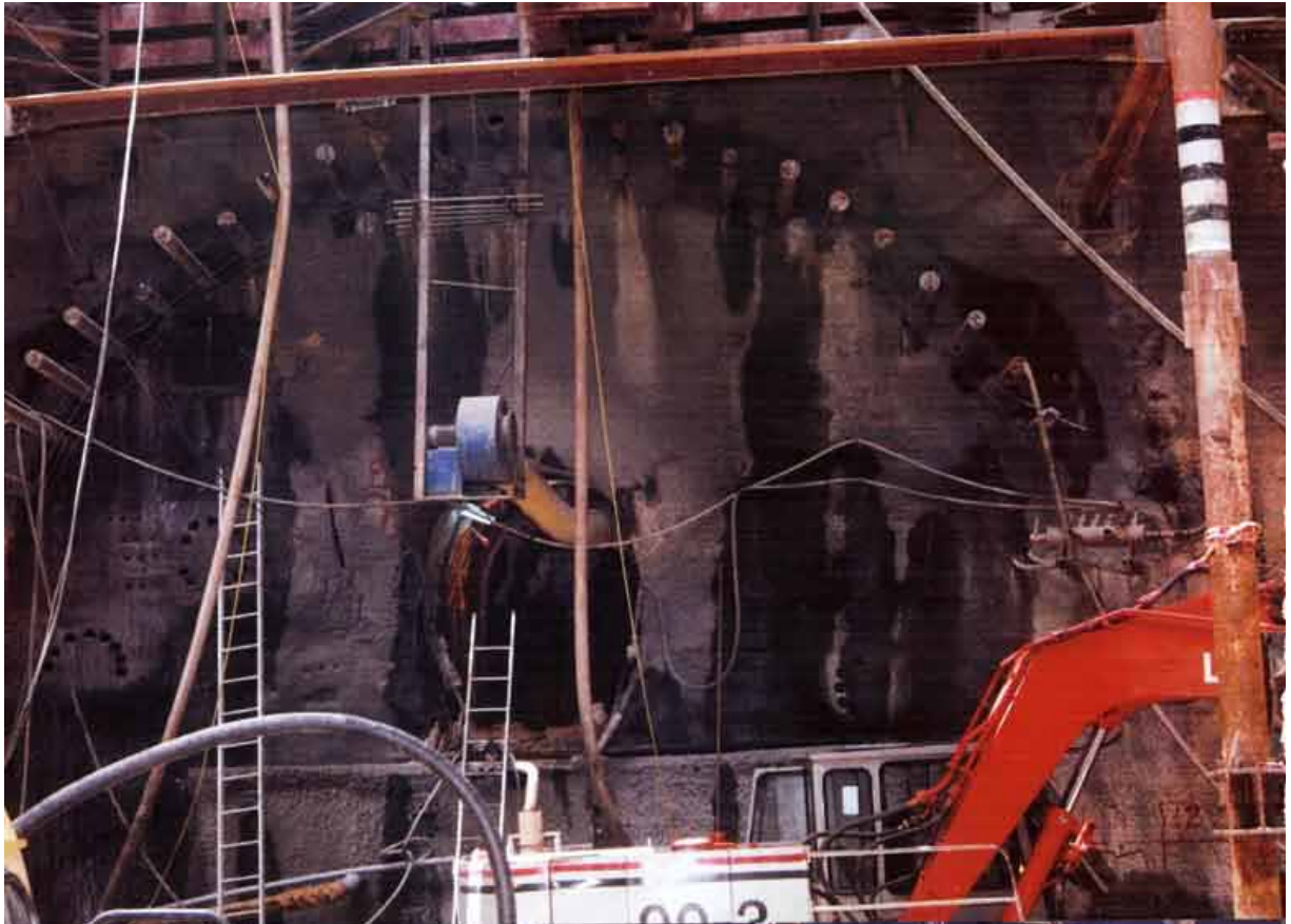
Pipe Roofing at Amar Cinema Shaft, MC1B, Delhi Metro Rail Corporation, New Delhi, India
